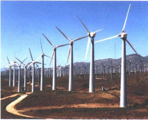
Wind turbines at Tehachapi Pass, California. Photo courtesy of the U.S. Department of Energy.
